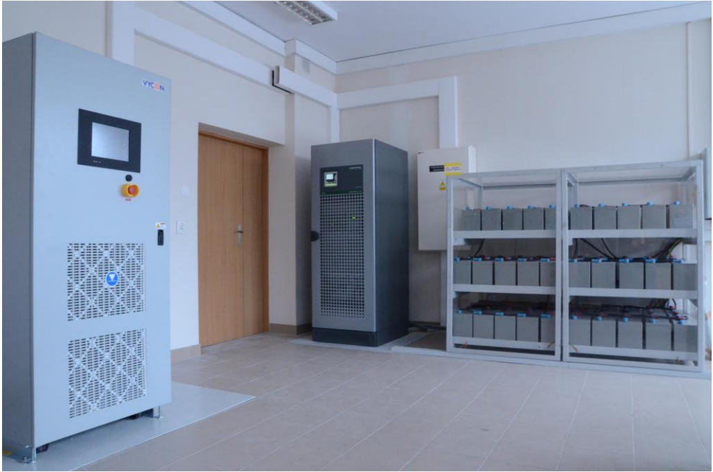
Photograph: Vycon Flywheel 350 kW and Socomec UPS 160 kVA system with battery stand (DER laboratory at TU Lodz)
