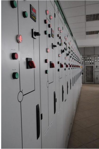
Photograph: Switching panel of the micro grid testing facility (DER laboratory at TU Lodz).
