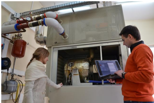
Photograph: Microturbine system Capstone C30 (DER laboratory at TU Lodz)
